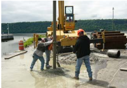
Saw Mill River Bridge, Yonkers, NY Piles to support new bridge structure.
